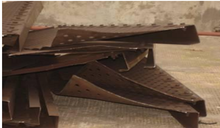
Figure 9 Damaged trays of the 433-V4 Toluene Column
