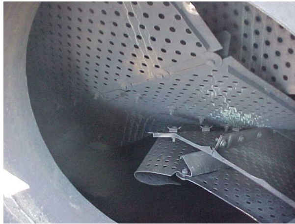
Figure 3 Tray damaged and collapsed from upper section to middle section of 100-V3 (Nov. 2000)
